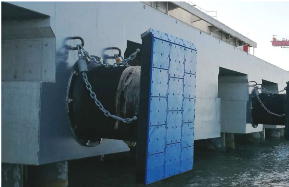
舟山港衢山港区鼠浪湖矿石中转码头 TD-A2500×1×1 橡胶护舷安装实例 Shulang Lake Ore Transfer Terminal, Qushan Port Area, Zhoushan Port
