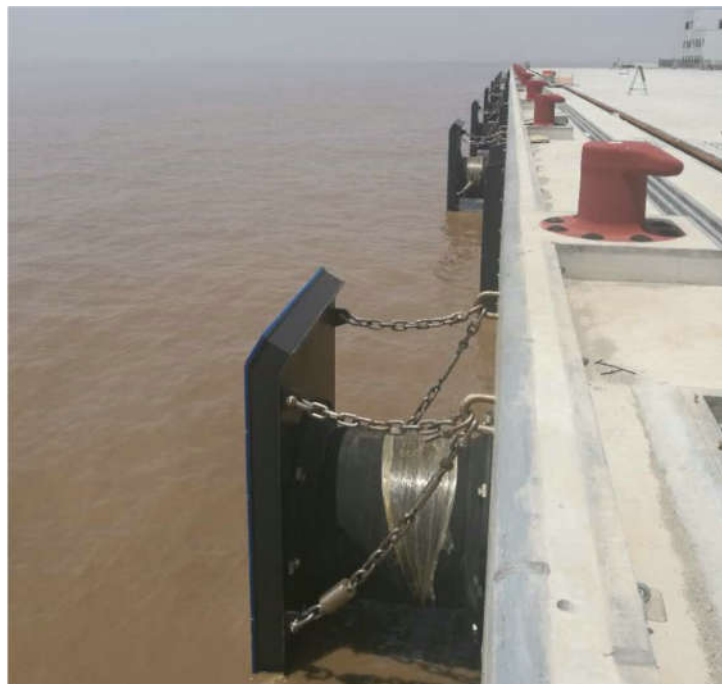
洋山深水港四期项目橡胶护舷安装实例 Installation of Rubber Fender In Shanghai Yangshan Deepwater Port Phase IV Project
